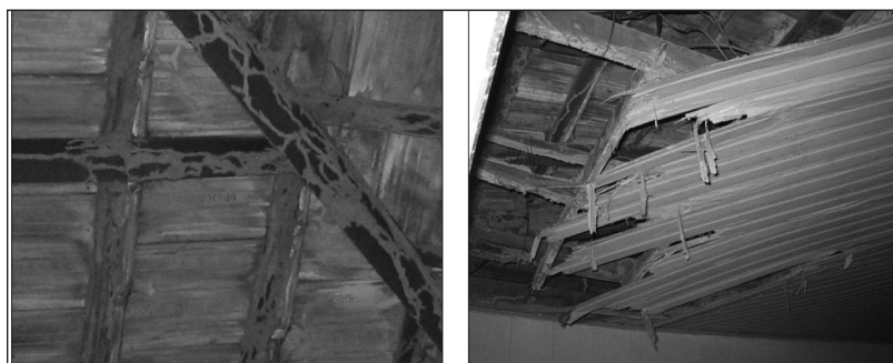
Photographs 1, 2. Tunnels of subterranean termites in roof structure; ceiling damaged by termites (Photos: File IPT)
